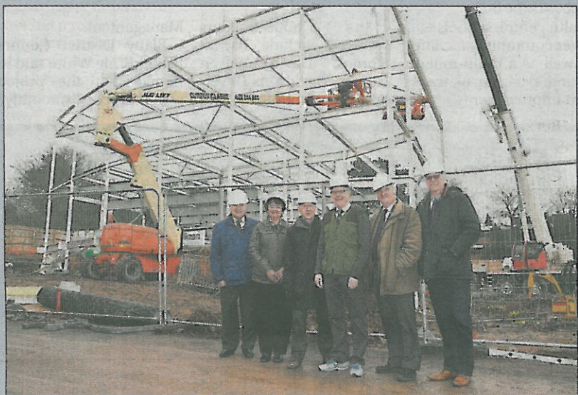
Start of construction work on Hinckley's new leisure centre. Left to right, Cllr Rob Mayné, Cllr Bron Witherford, the Mayor of Hinckley and Bosworth, Cllr Jeff Bannister, Cllr Bill Crooks, Cllr David Bill and Cllr David Cope. Picture: Matt Buchan
