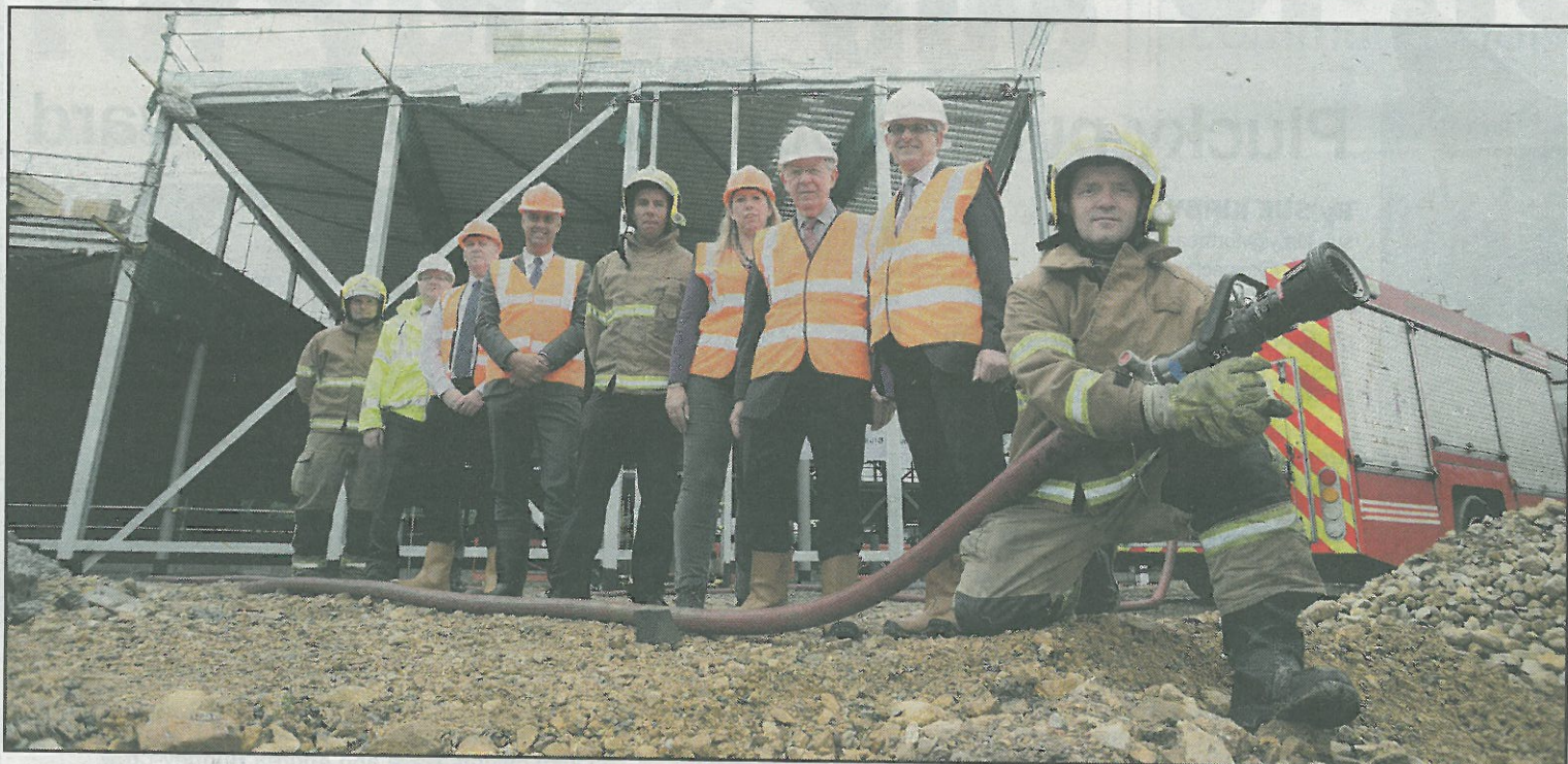
ALL SET: Left to right ... Firefighter Ian Haskell, Ian Parkin, Craig Jobson, Jan Peeters, Neil Burnett, Cllr Dianne Snowdon, Cllr Harry Trueman, Dave Smith and Firefighter Bob Foster pictured before spraying water into the new Washington Leisure centre swimming pool for the first time today
