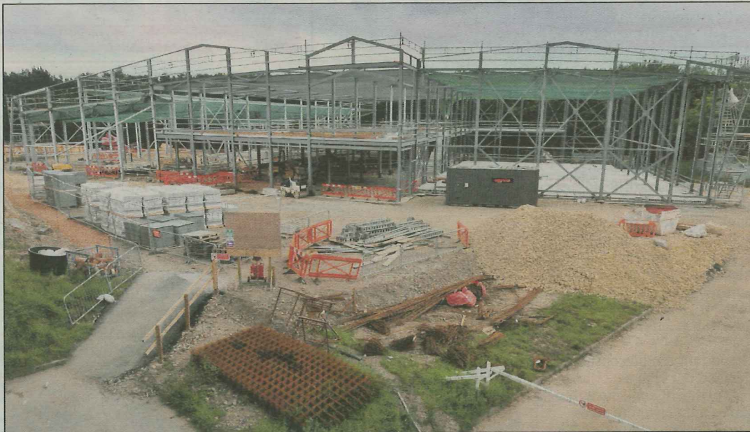
TAKING SHAPE: The new Washington Leisure Centre, which is being built behind the old facility.
